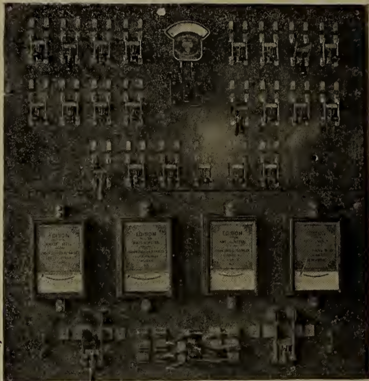
SWITCHBOARD, HOTEL REGENT, BROOKLYN, N. Y.
