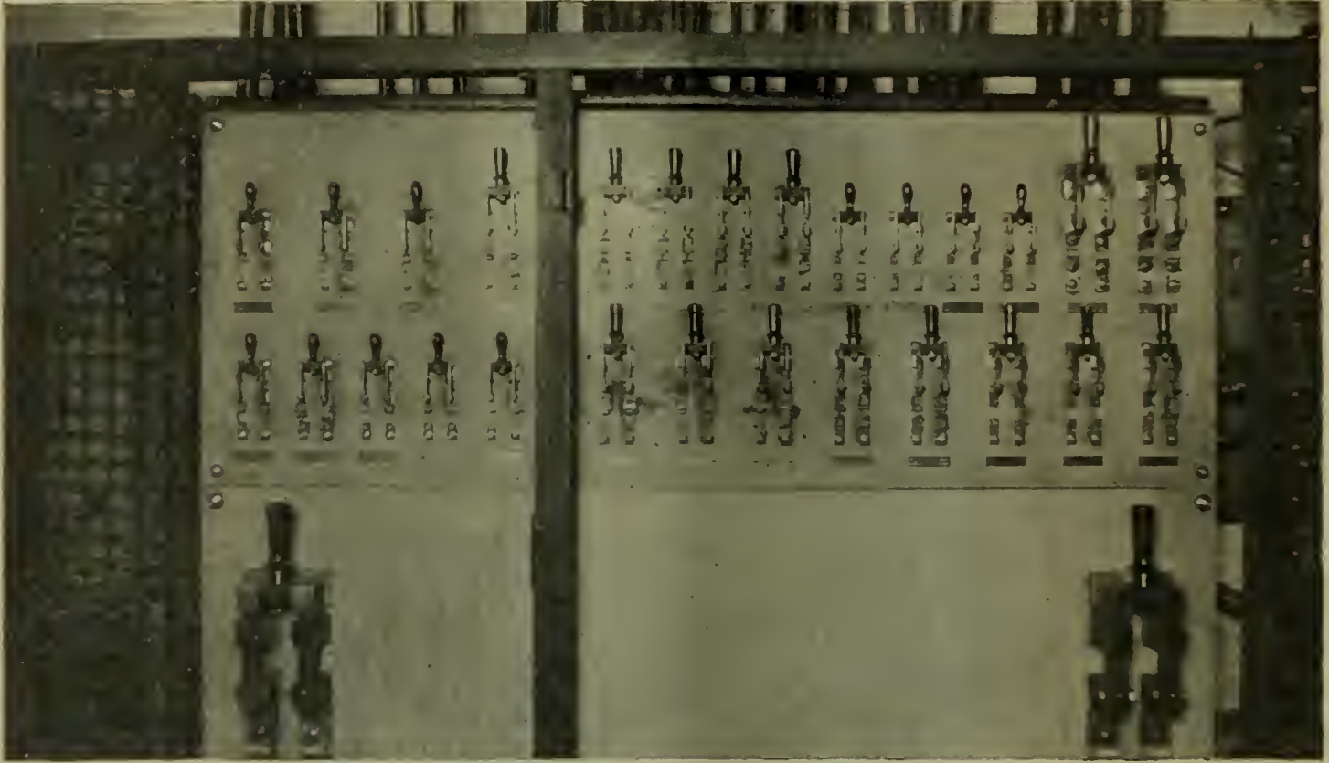
Switchboard. Garvin Machine Co.
