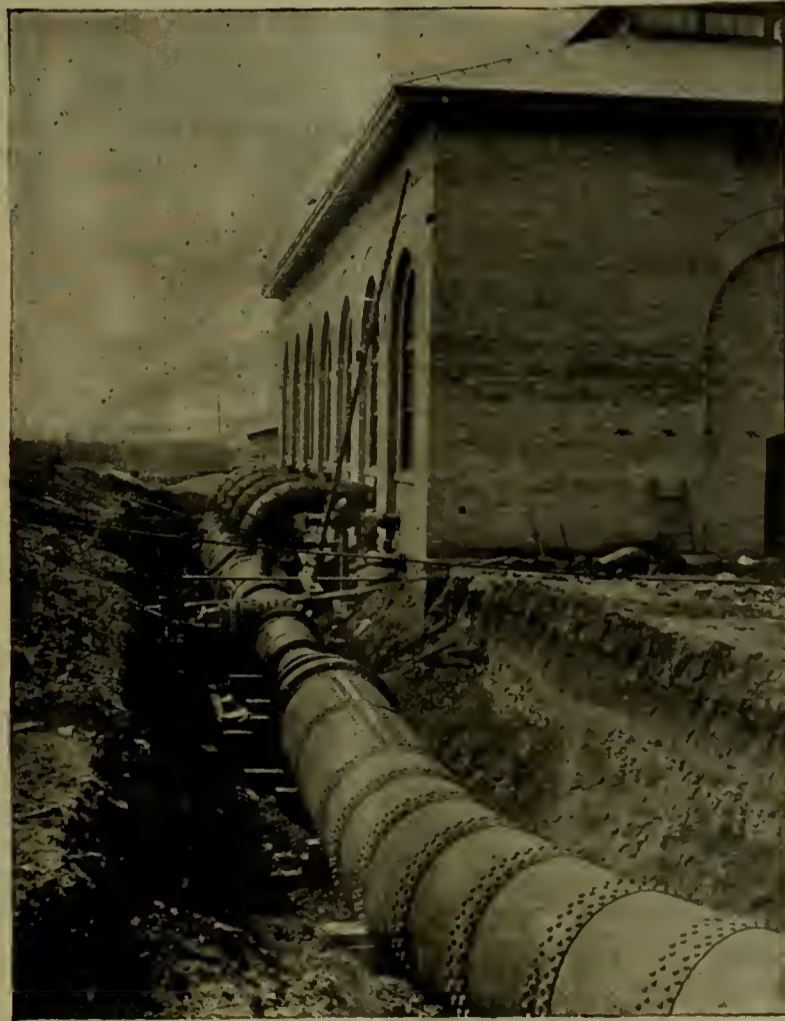
Fig. 4.—Exterior of Power House, Showing one Venturi Motor and Receiver.
