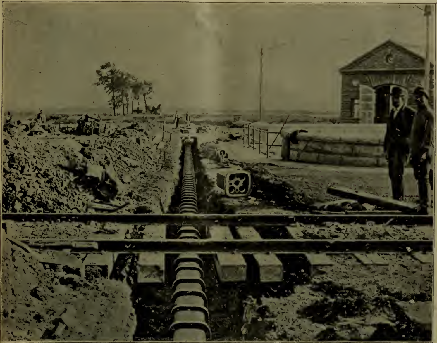
Showing construction of Tellmic Conduit to convey Electrical Power from The Cataract Construction Co.'s Colossal Electrical Generating Plant at Niagara Falls, New York, the greatest electrical power in the world carried underground.
