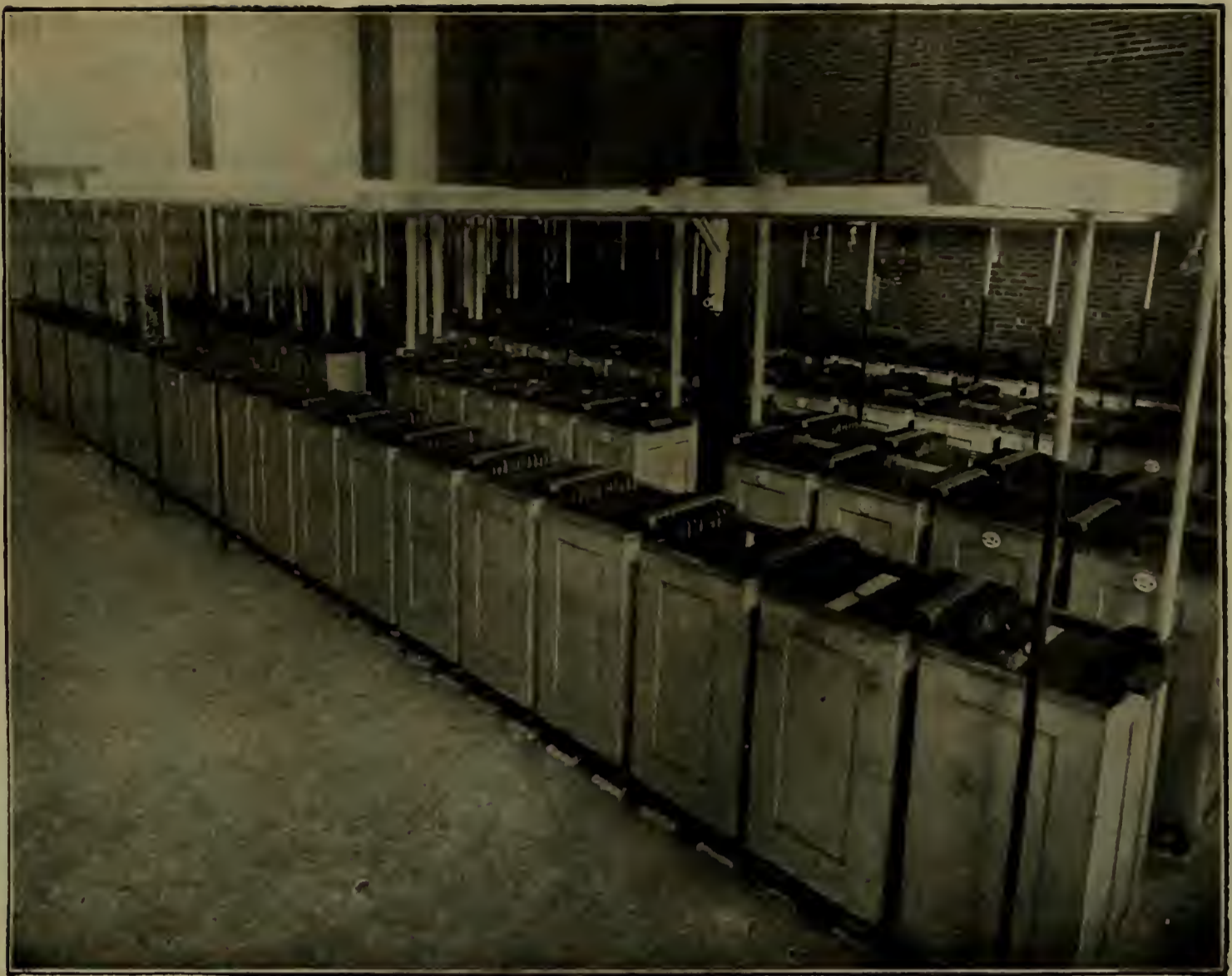
Boston Edison Station. The First Independent Battery Station in America of Chloride Accumulators.
