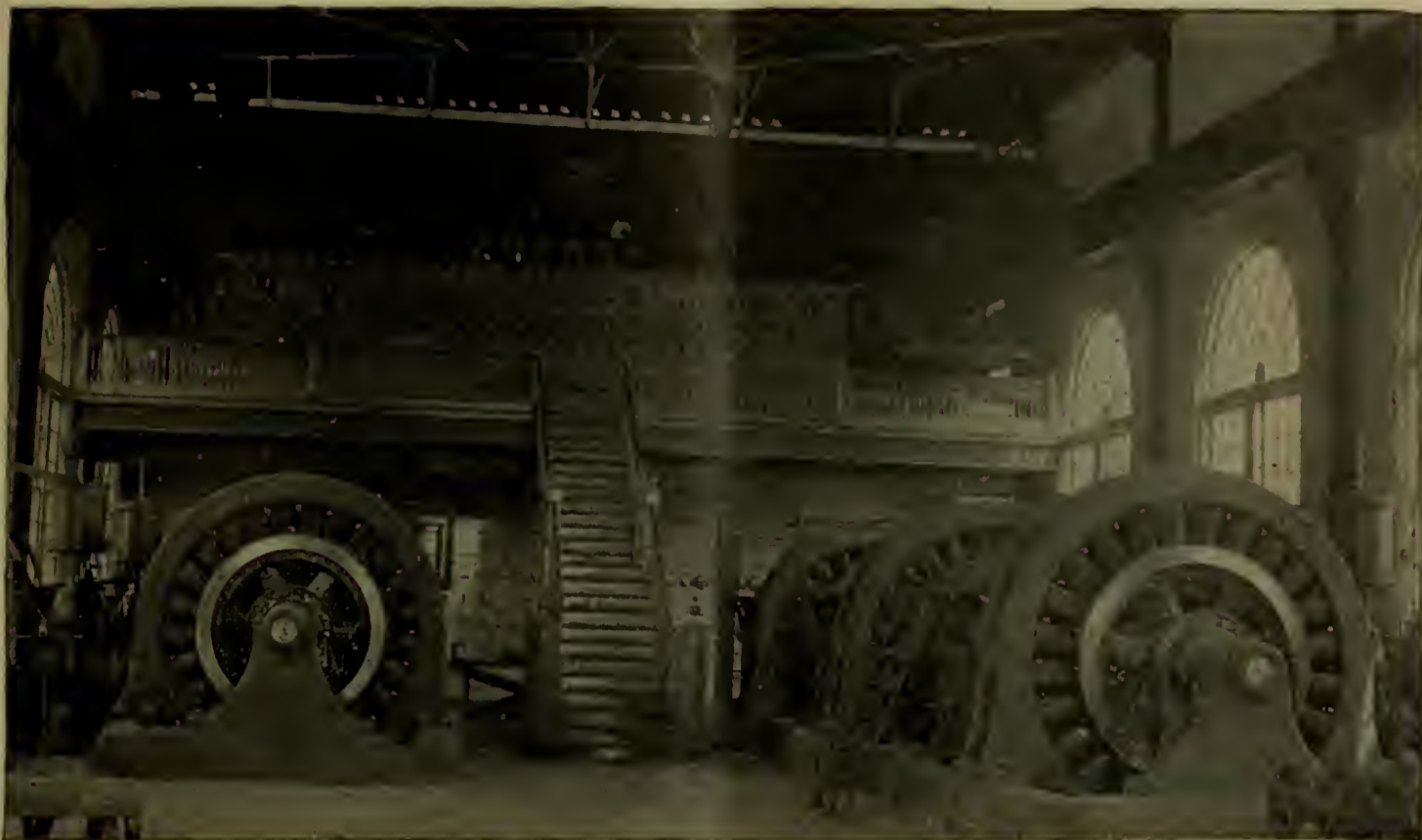
Fig. 7.—Interior of Power House.
