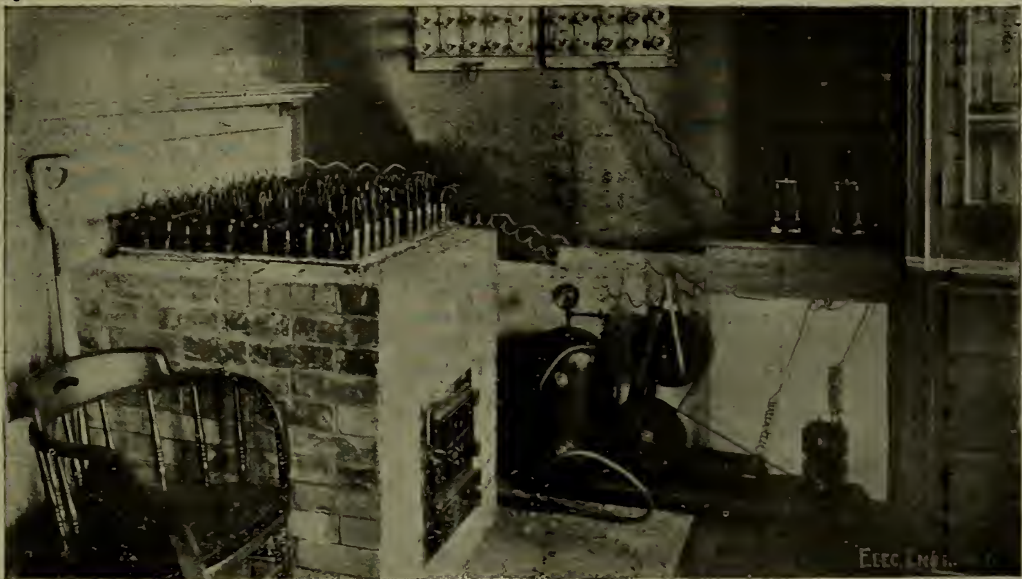
The Jacques Battery in Operation.
