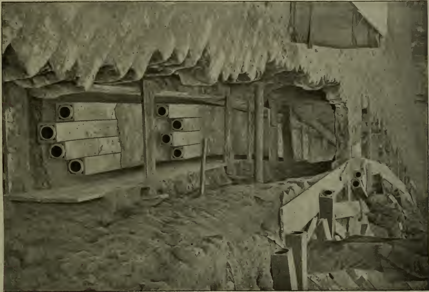
Conduits Illustrating Curved Construction.
