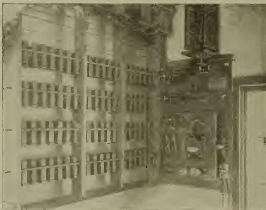
Small Storage Battery Installation.
