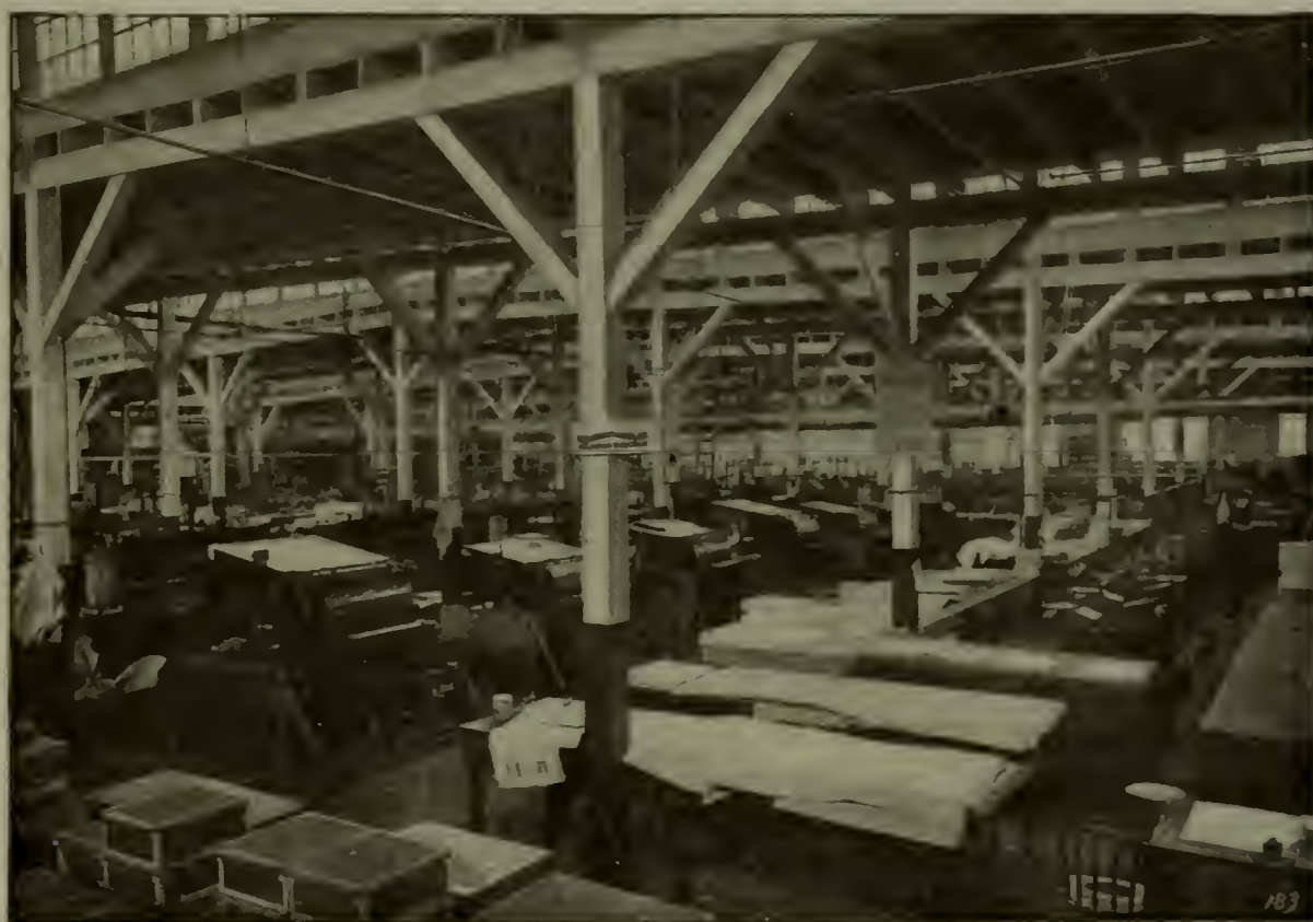
Printing Room Showing Electrically Driven Presses and Absence of Belting and Shafting; 45 C. W. Motors Installed in this Room.
