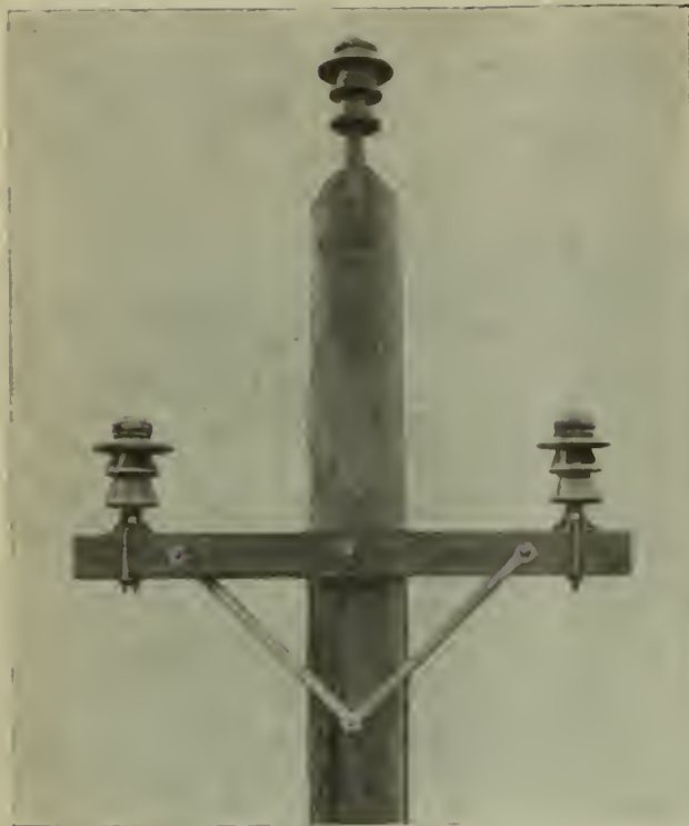
Fig. 10. DETAILS OF POLE TOP, 44,000 VOLTS.
