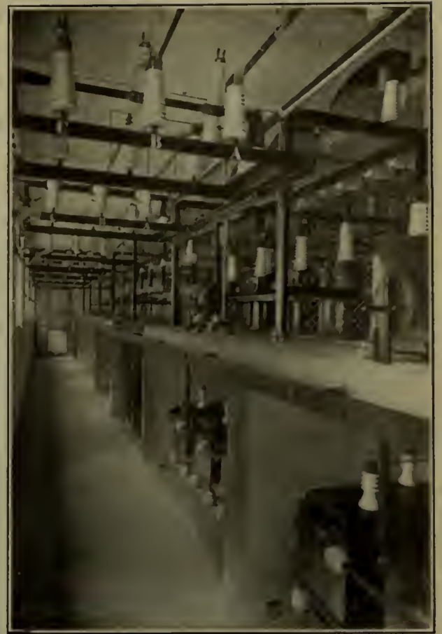
Fig. 10.—35,000-VOLT BUS-ROOM, SHOWING ALSO MOTOR-ACTUATED OIL SWITCHES, HEIMBACH PLANT, GERMANY.
