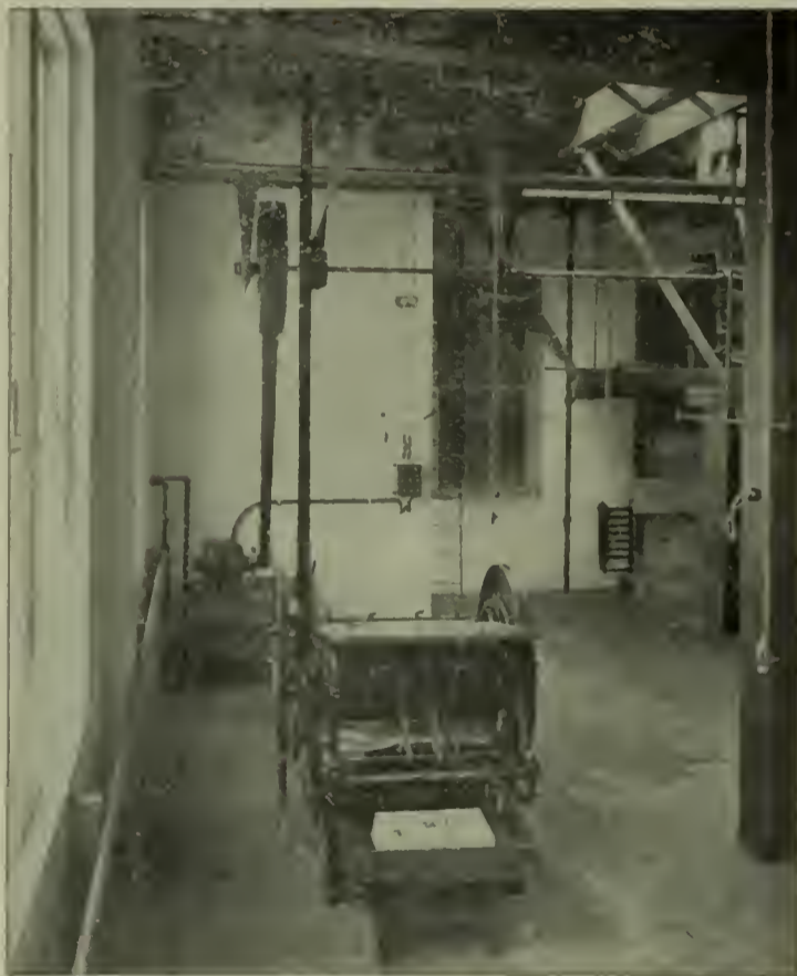
FIG. 5.—5 H.P. 220 VOLT KG SINGLE-PHASE MOTOR DRIVING LINE SHAFTING, FROM WHICH ARE DRIVEN CUTTING PRESSES AND SPECIAL MACHINES USED IN SHAPING AND FINISHING, AND THE DRIVING PRESS SHOWN IN THE FOREGROUND. NOTE THE NEAT JOB OF WIRING AT THE MOTOR.
