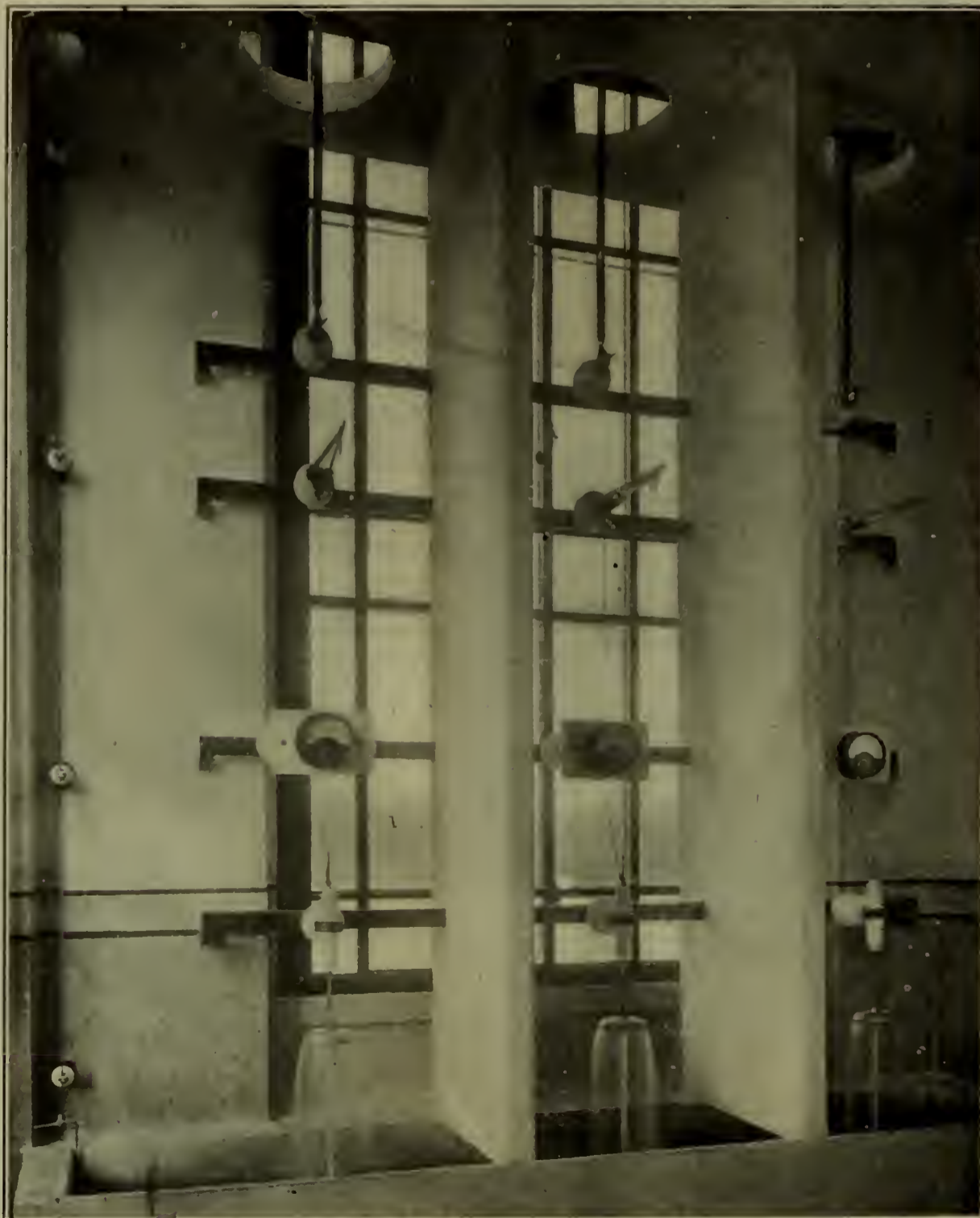
Fig. 15.—50,000-VOLT WATER-FLOW GROUNTERS AT THE STEP-UP STATION, PIATTAMALA, ITALY.
