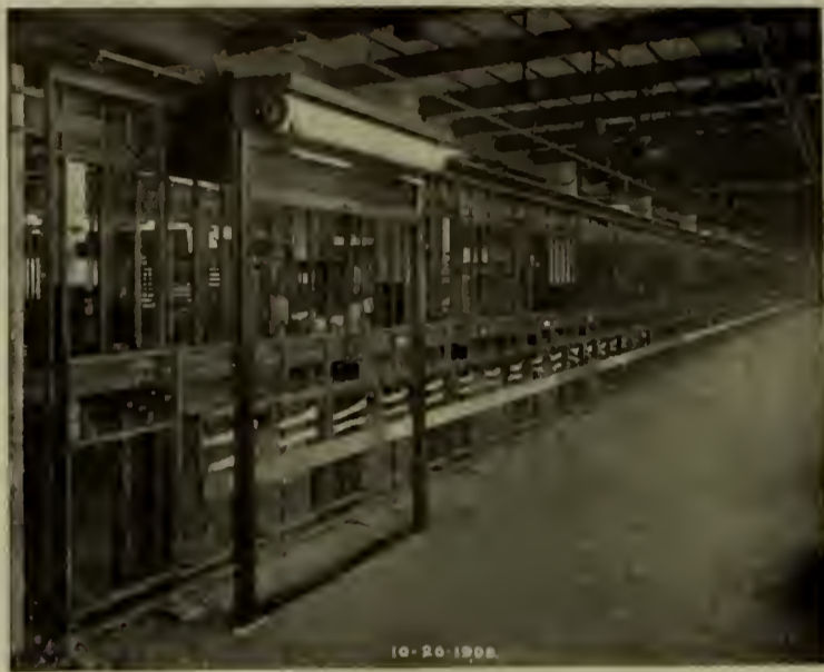
REAR VIEW OF TELEPHONE SWITCHBOARD, SHOWING FRAMEWORK.
