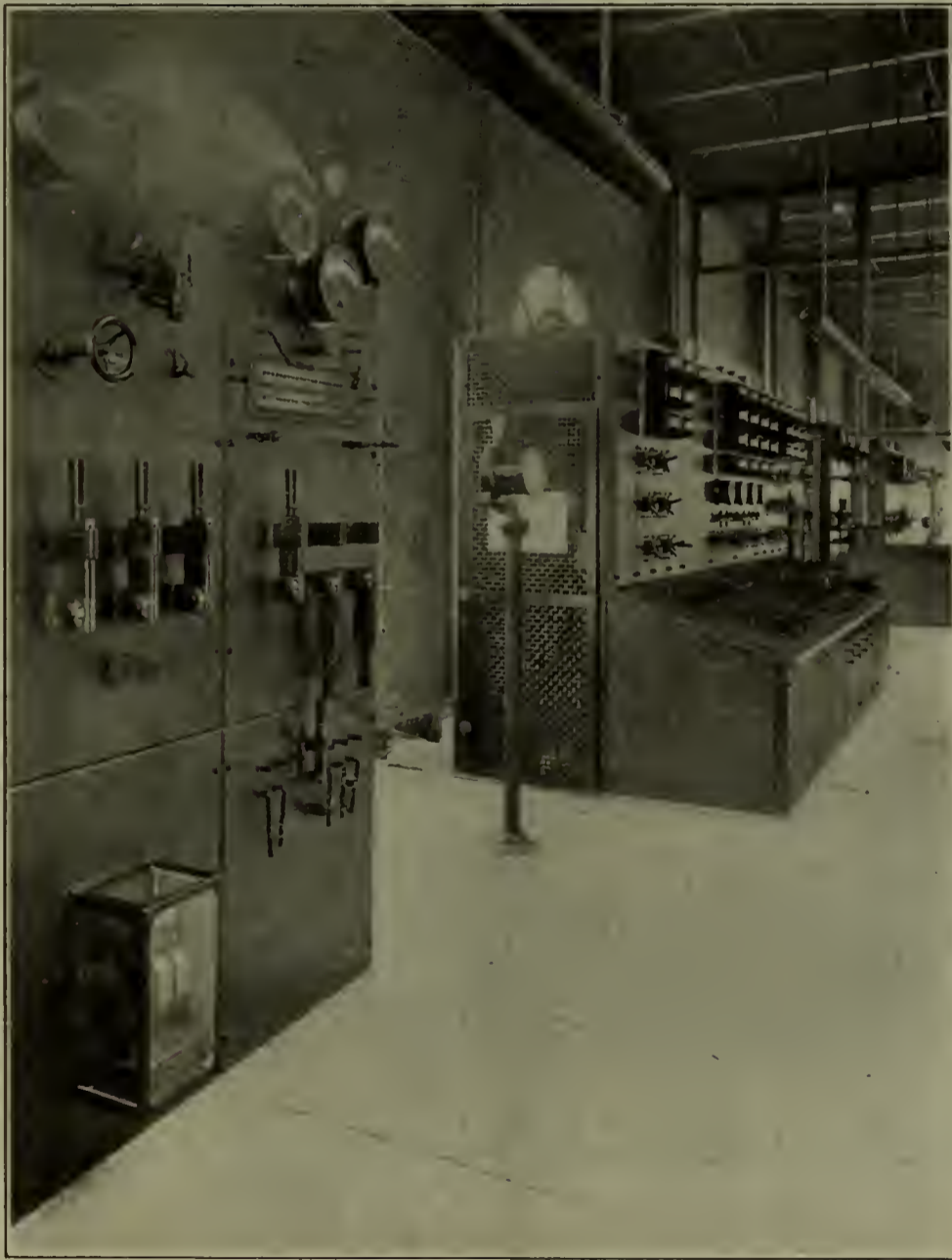
FIG. 7.—CONTROL DESK WITH HORIZONTAL EDGEWISE METERS, NEW YORK CENTRAL AND HUDSON RIVER RAILROAD, PORT MORRIS POWER STATION, NEW YORK.
