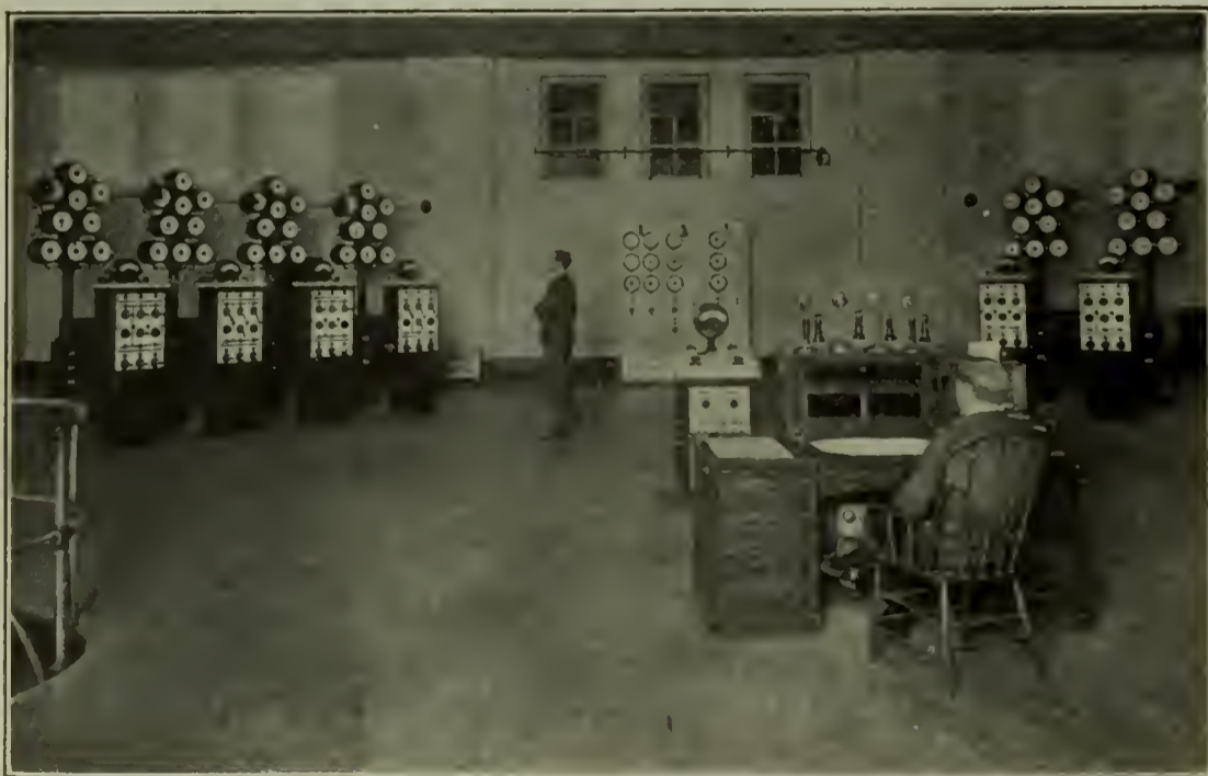
FIG. 5.—CONTROL ROOM WITH PEDESTALS AND POSTS, ONTARIO POWER CO., NIAGARA FALLS, CANADA.
