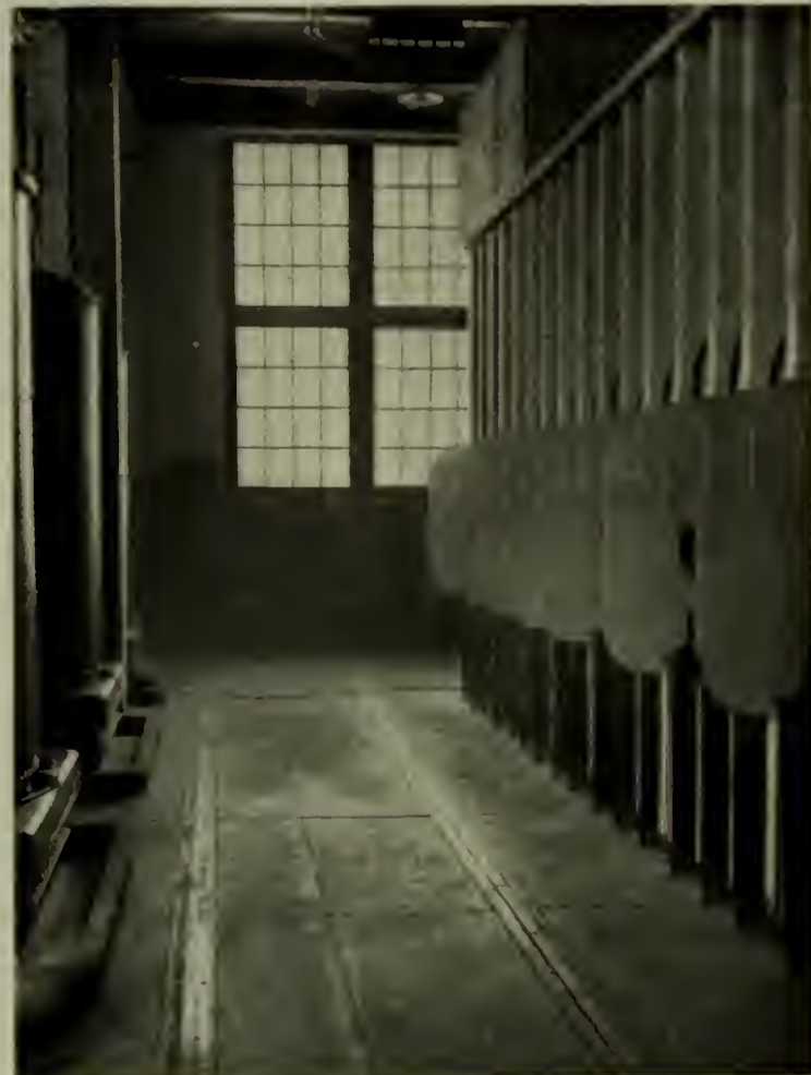
Fig. 6. AISLE BETWEEN SWITCH STRUCTURE AND TRANSFORMERS.
