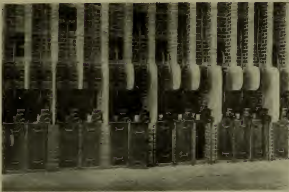
Fig. 7. OIL SWITCHES AND BUS STRUCTURE.
