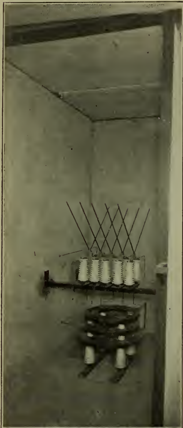
Fig. 13.—SIEMENS-SCHUCKERT HORN GAPS, WITH CHOKE COILS, HEIM 35,000-VOLT PLANT, GERMANY.
