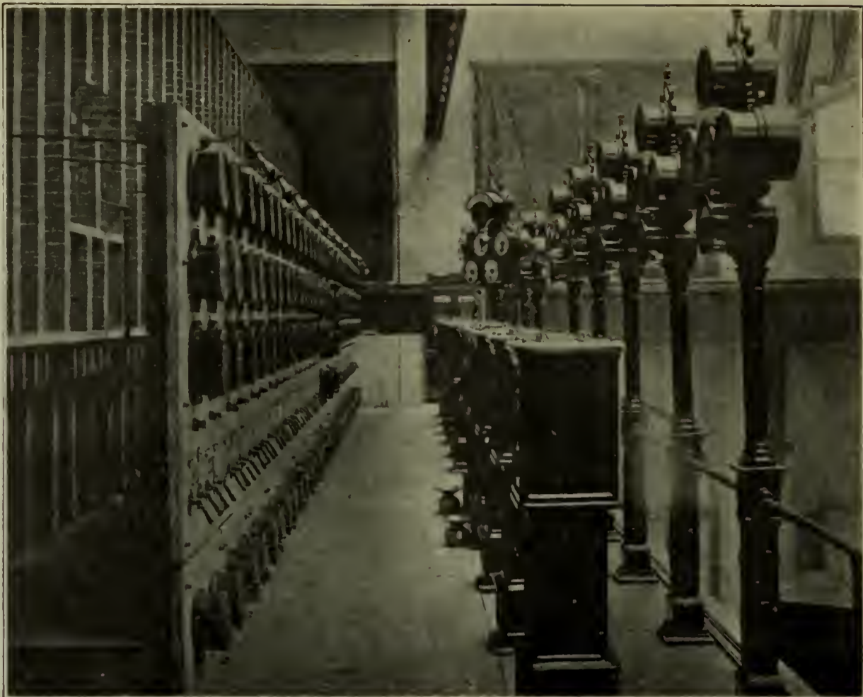
FIG. 4.—GALLEY WITH PEDESTAL POSTS FOR UNION ELECTRIC LIGHT & POWER CO., ST. LOUIS.
