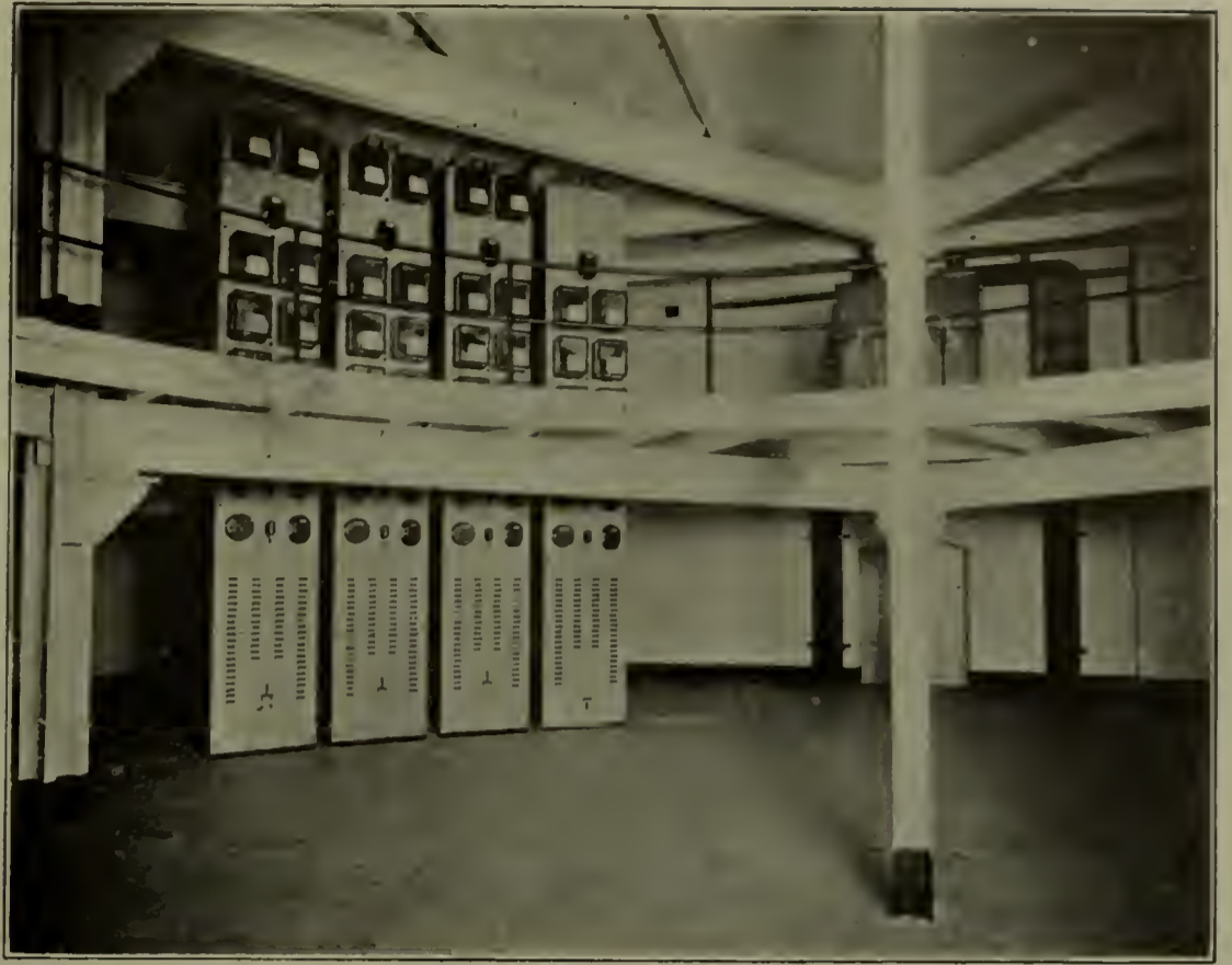
FIG. 6.—SWITCHBOARD GALLERIES SHOWING TERMINAL, RELAY AND RECORDING INSTRUMENT BOARDS, ONTARIO POWER CO., NIAGARA FALLS, CANADA.
