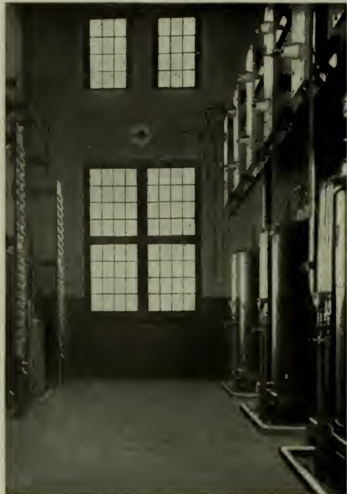
Fig. 5. AISLE BETWEEN TRANSFORMERS AND LIGHTNING ARRESTERS.
