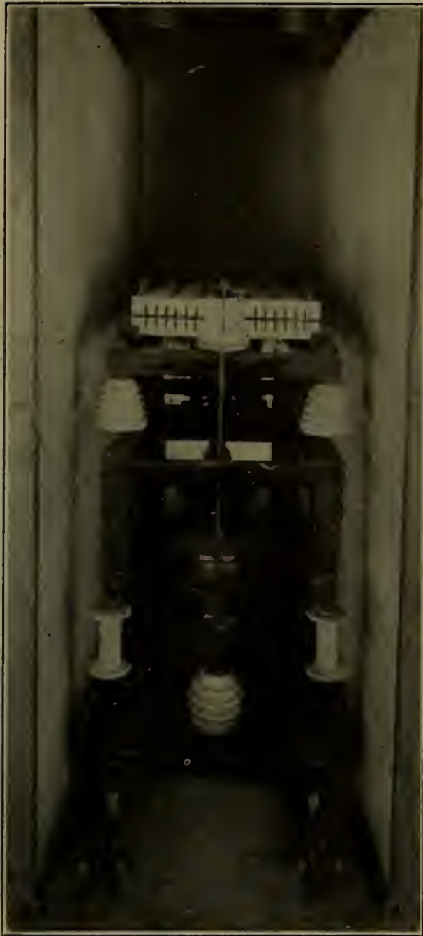
Fig. 16.—BROWN, BOVERI MULTIGAP LIGHTNING ARRESTER CONNECTED TO WATER RHEOSTAT, LOFUTCH PLANT, SWITZERLAND.
