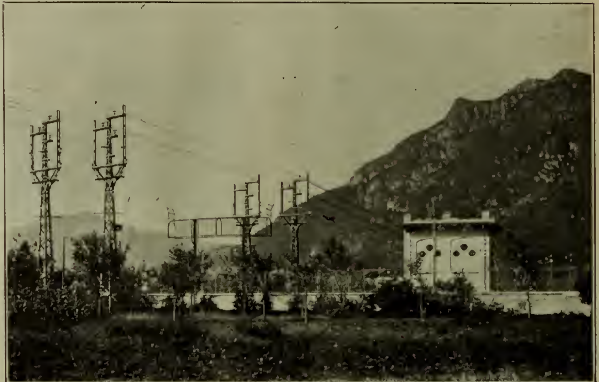
Fig. 20.—HIGHWAY AND TELEPHONE CROSSING OF 50,000-VOLT LINE NEAR LECCO, ITALY, ALSO SECTION SWITCH-HOUSE.
