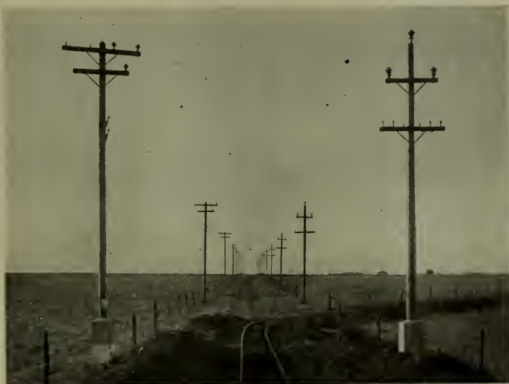
Fig. 9. MAIN TRANSMISSION LINES LEAVING POWER HOUSE.
