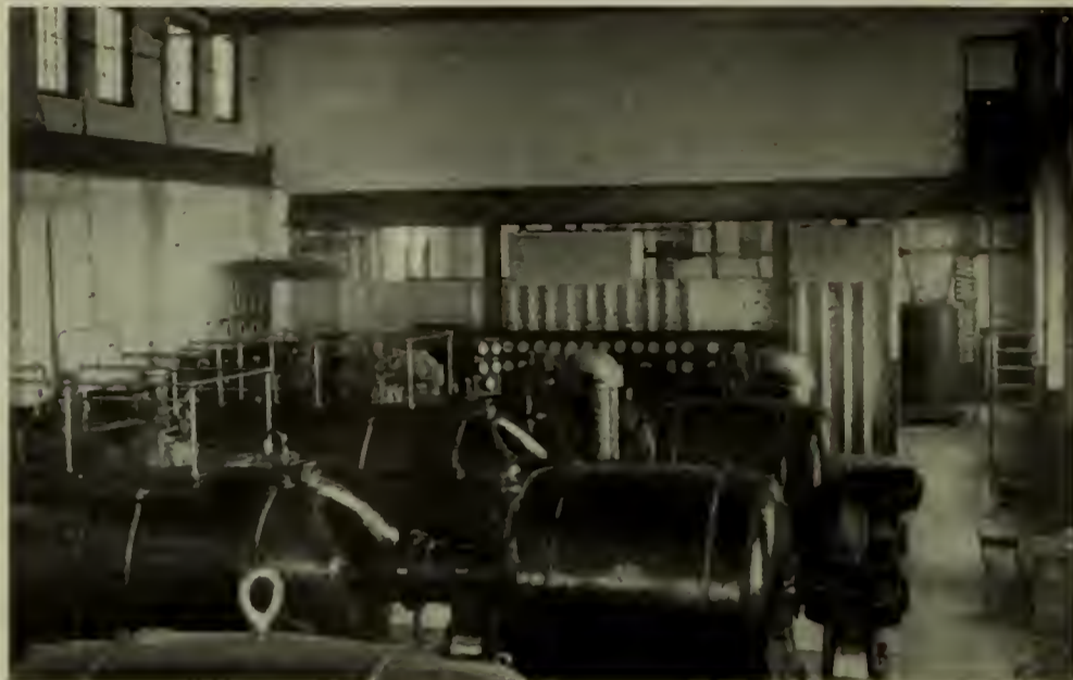
Fig. 4. TURBINE ROOM, SHOWING SWITCHBOARD IN REAR.
