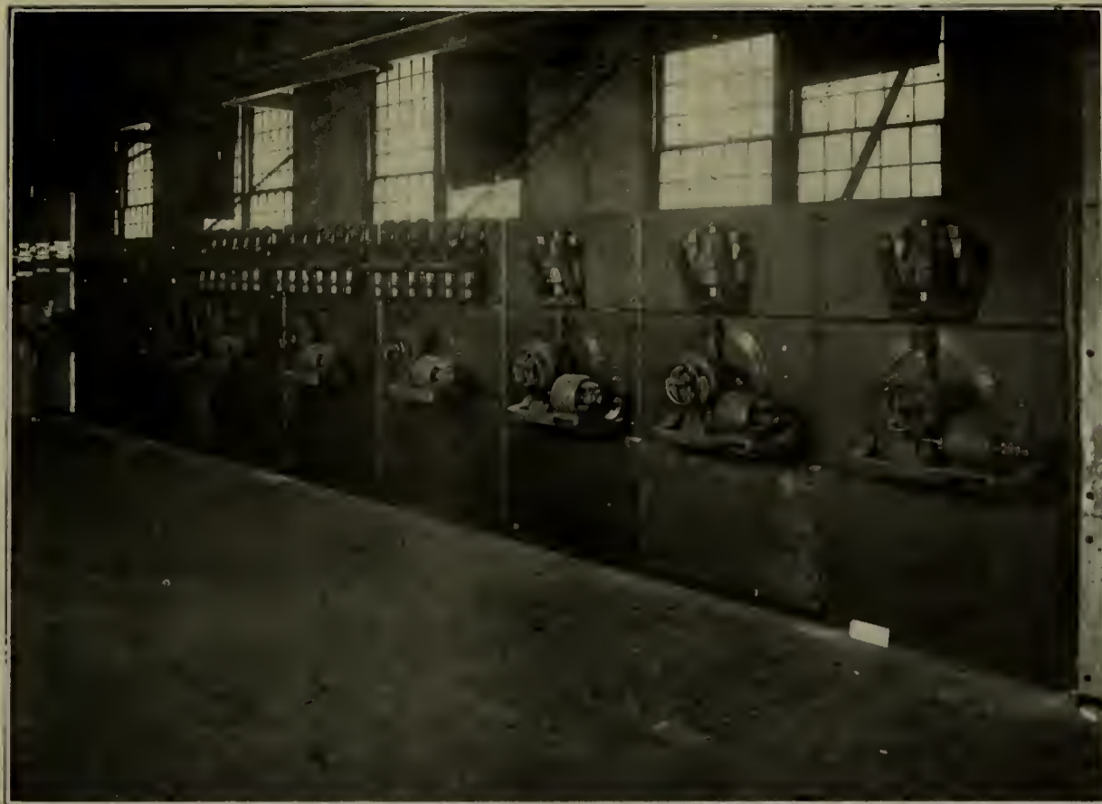
FIG. 11.—FIELD SWITCHBOARD, RIO JANEIRO TRACTION, LIGHT & POWER CO., RIO JANEIRO, BRAZIL.
