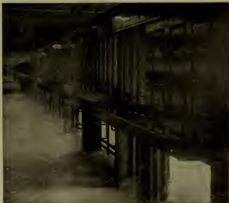
FRONT VIEW OF SECTION OF NEW WESTERN ELECTRIC PARIS TELEPHONE SWITCHBOARD.
