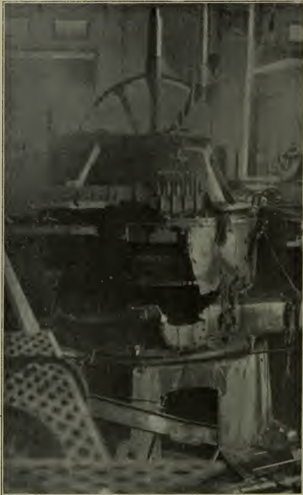
2000-KW. VERTICAL TURBO-GENERATOR IN STATION OF CALIFORNIA GAS & ELECTRIC CO., LOS ANGELES, CAL.
