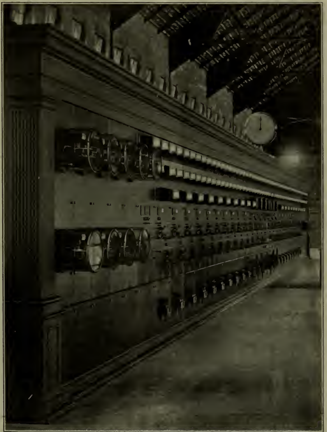
FIG. 2.—PANEL SWITCHBOARD HORIZONTAL EDGewise METERS FOR CANADIAN NIAGARA POWER CO., VIEW OF NO. 1 SWITCHBOARD.
