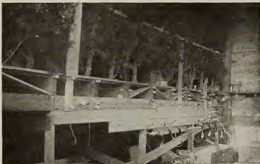
The Extemporized Switchboard: Simple but Sufficient
