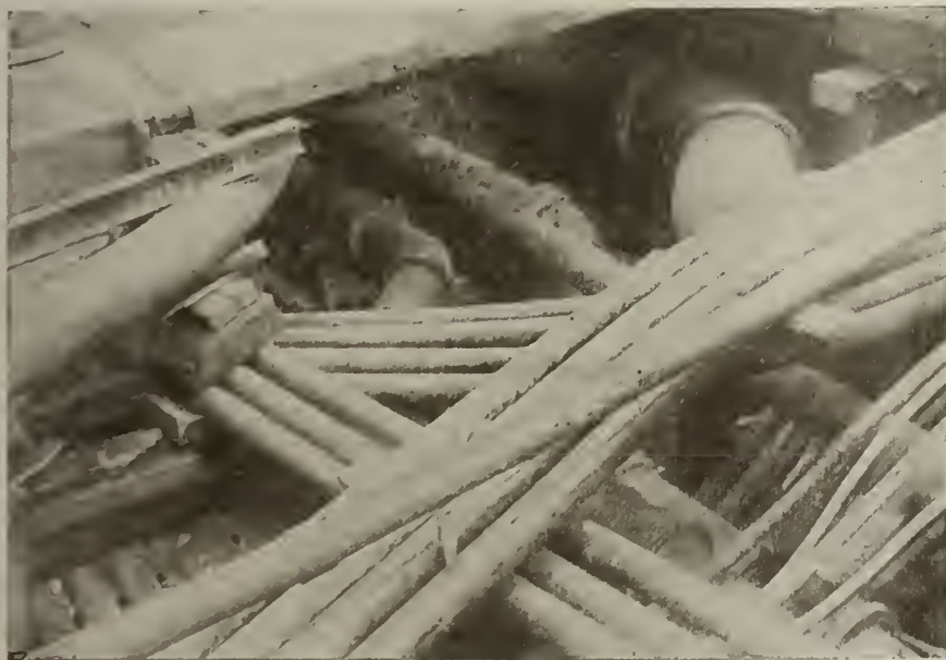
S. E. Corner Broadway and Pearl Streets, Empire City Pipe Ducts on Top.
