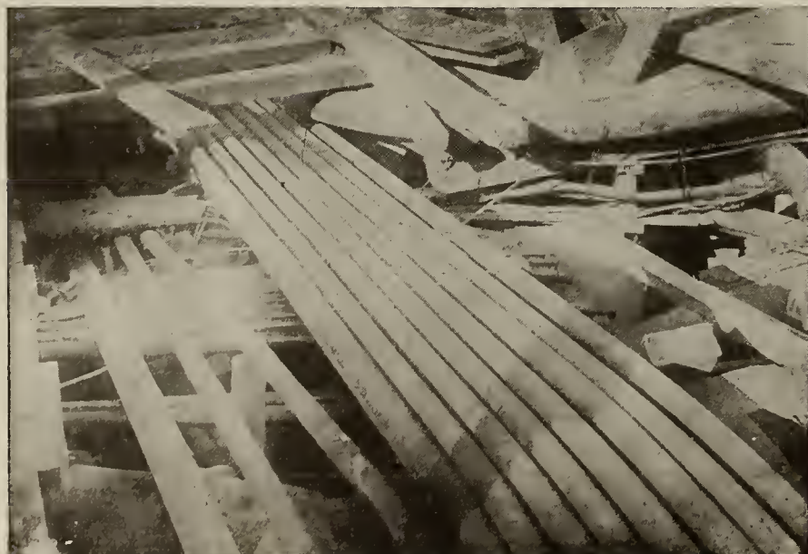
S. E. Corner Broadway and Canal Streets. 24-duct subway above; 16-duct below.
