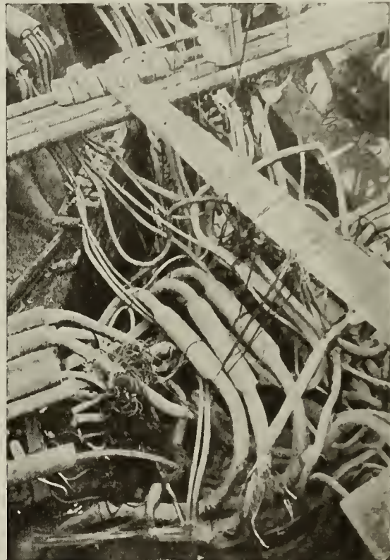
S. E. Corner Broadway and Houston Streets. Telephone Cables Exposed During Reconstruction of Manhole.
