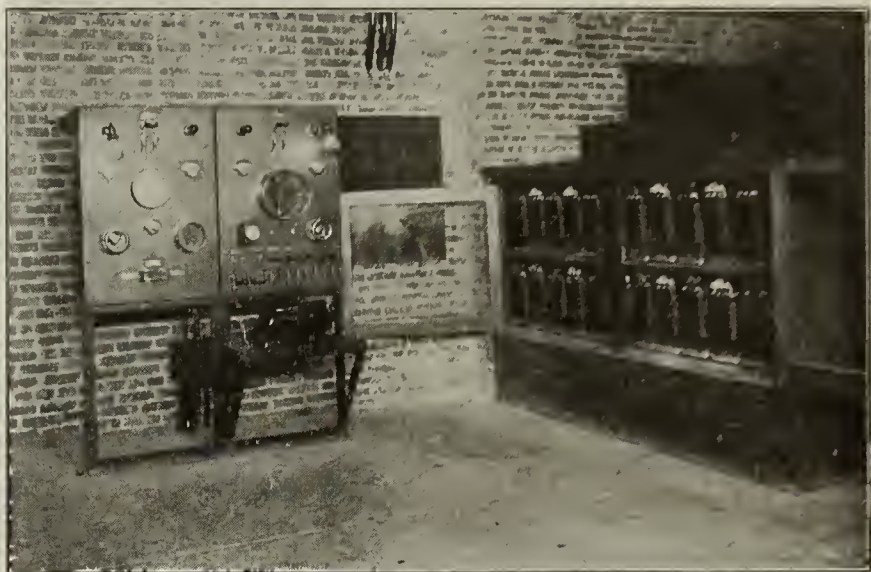
Low-voltage Switchboard and Battery
