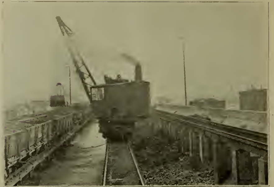
LOADING CINDERS WITH CRANE. THE CINDER PIT FULL OF WATER IS SHOWN. COAL STORAGE BINS ON RIGHT—LOCOMOTIVE TERMINAL AT CHICAGO, C. & W. I. R. R.
