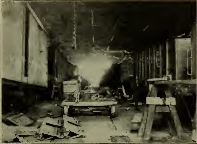
VIEW DOWN SERVICE TRACK IN STEEL CAR BAY.—FREIGHT CAR REPAIR SHOP, MC KEES ROCKS, PITTSBURGH AND LAKE ERIE R. R.
