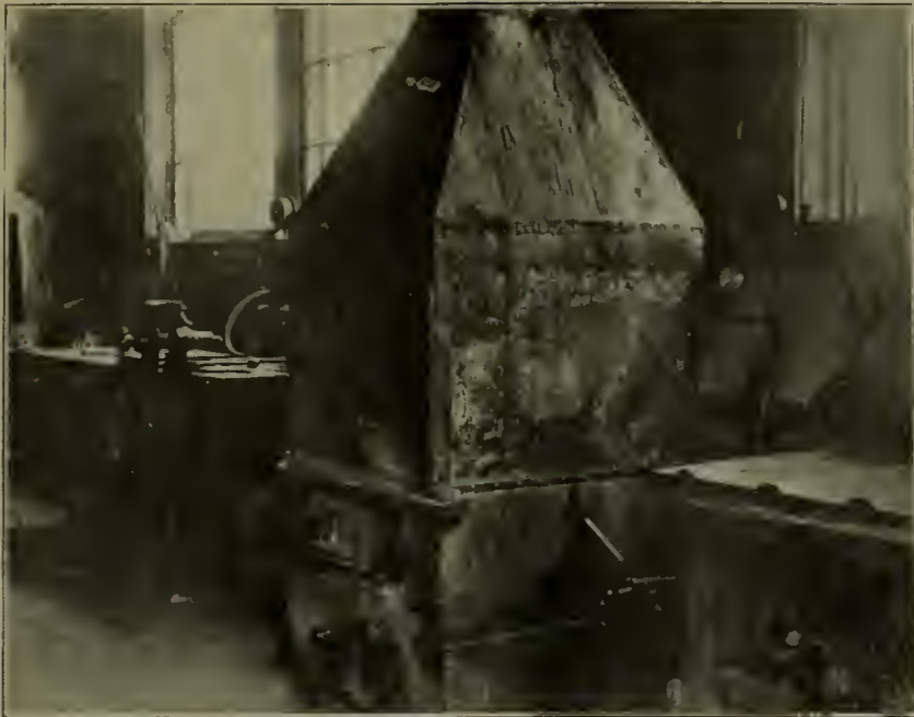
FERGUSON FURNACE FOR MELTING BABBITT IN TIN SHOP—CAR REPAIR SHOP AT EAST DECATUR, WABASH RAILROAD.
