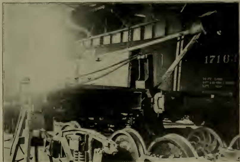
ILLUSTRATING THE CLASS OF REPAIRS MADE TO STEEL CARS. NATURAL GAS BURNER BEING USED TO STRAIGHTEN SIDE ANGLES.—FREIGHT CAR REPAIR SHOP, MC KEES ROCKS, PITTSBURGH AND LAKE ERIE R. R.
