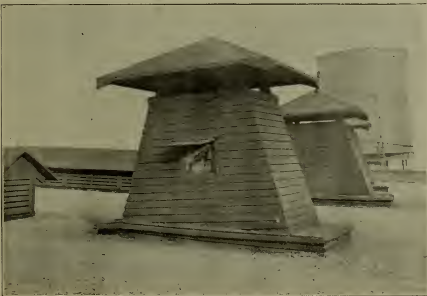
UPPER END OF SMOKE JACKS AND VENTILATORS ON THE ROOF OF ROUNDHOUSE—LOCOMOTIVE TERMINAL AT CHICAGO, C. & W. I. R. R.
