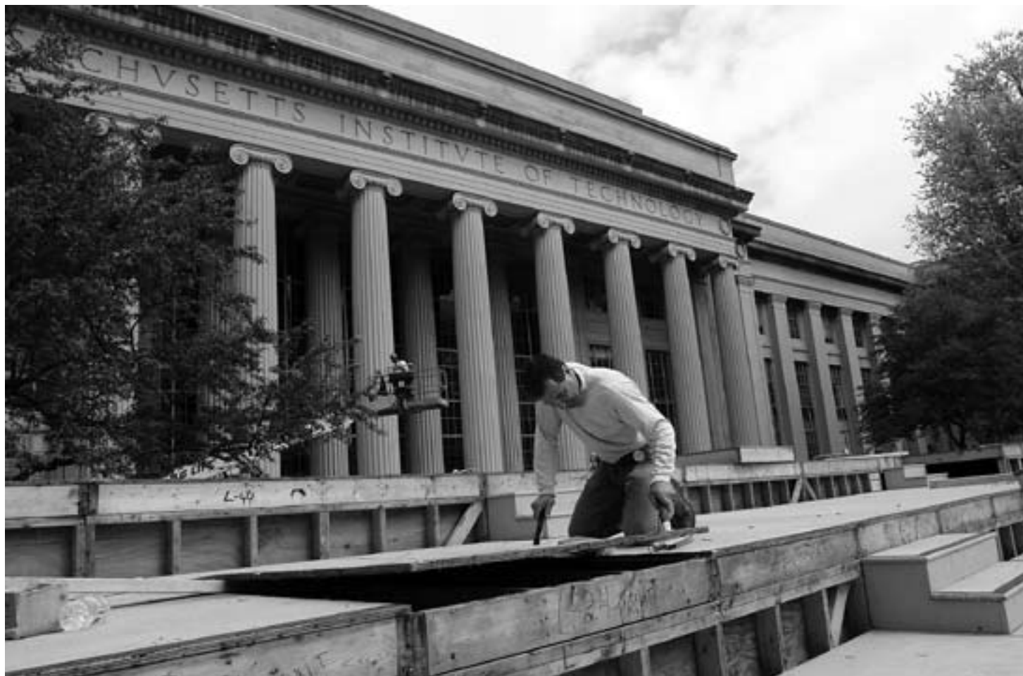
ABOVE: Facilities carpenter Rick Hodge checks and replaces old wood in the Commencement platform in preparation for graduation on June 6.
